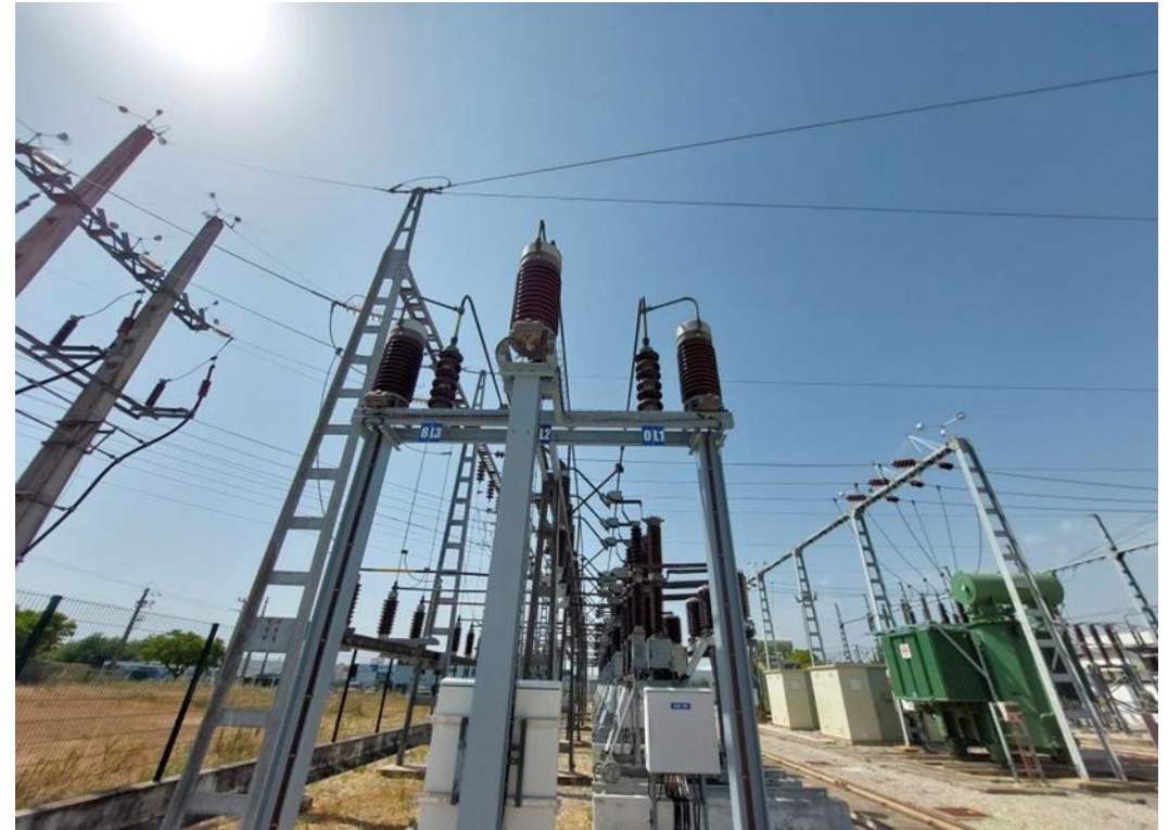
Figure: Almeirim substation: components from inside the substation.
