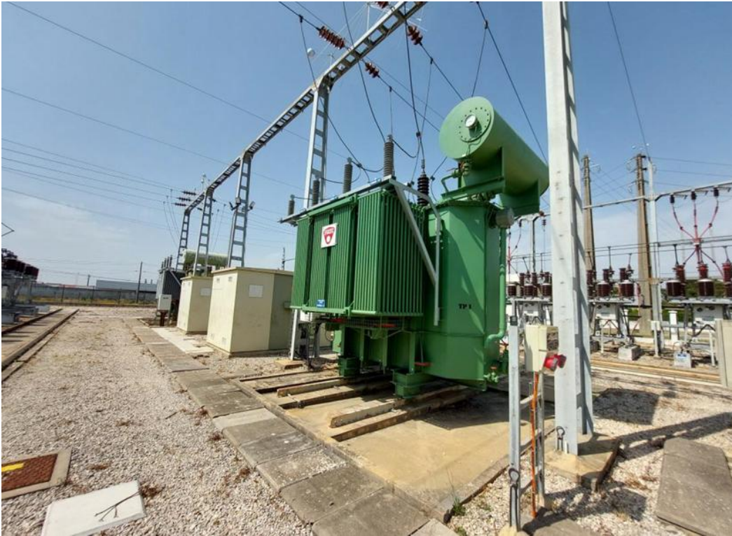
Figure: Almeirim substation: components from inside the substation.
