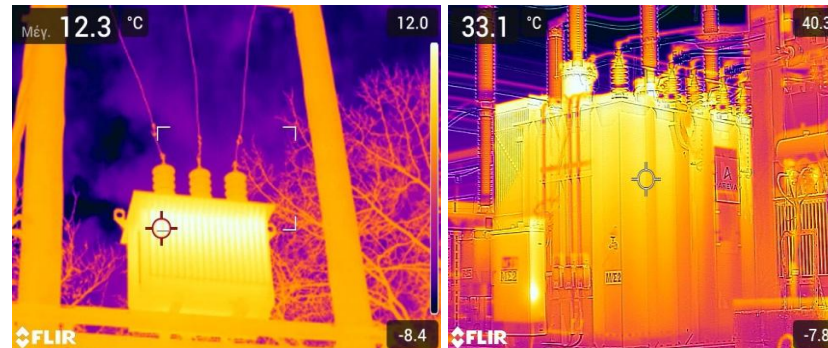
Thermal Images from Secondary/Primary Substations
